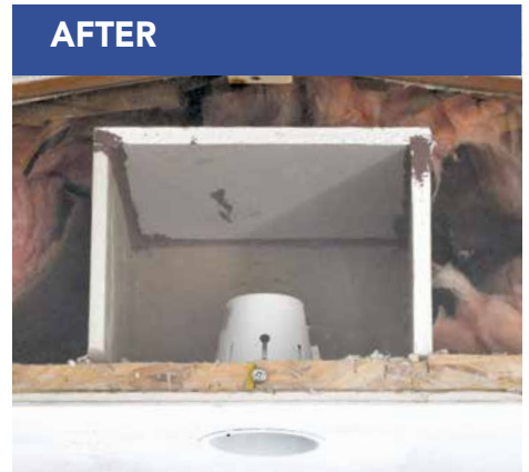
When boxed with appropriate clearances and fire-rated materials, fire risk is mitigated and air leakage is reduced.
