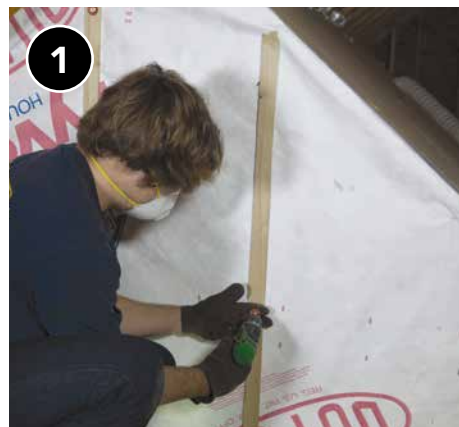
Securely install backing material over entire attic wall to create an enclosed cavity. Use wood strips along the studs and edges of the framing to hold the material in place, withstand air pressure, and prevent insulation from spilling out.
