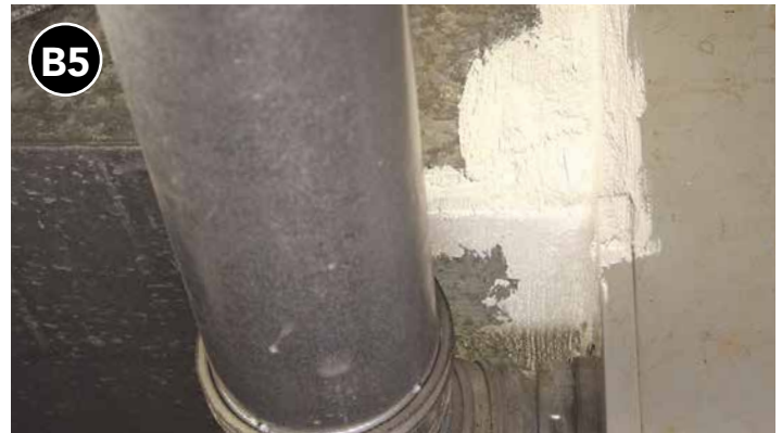
Apply additional mastic over mesh and tape, extending at least 1 inch past edges of tape in all directions.
