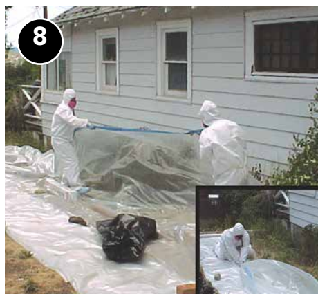
Clean work area and carefully fold and dispose of plastic sheeting in a plastic waste bag.
