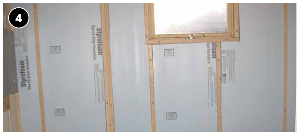
Install insulation using mechanical fasteners to prescribed R-value in full contact with the entire perimeter of the foundation wall from ceiling to floor.
