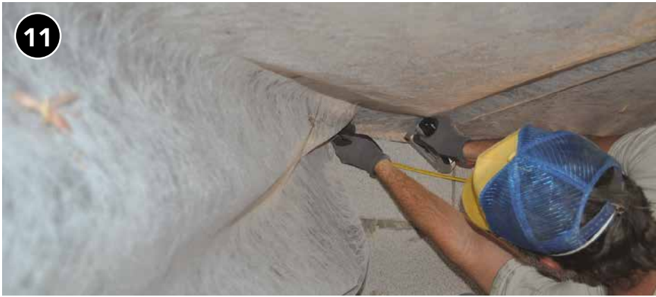
11 Cover the entire cavity to ensure continuous insulation coverage and prevent insulation from blowing out the ends.
