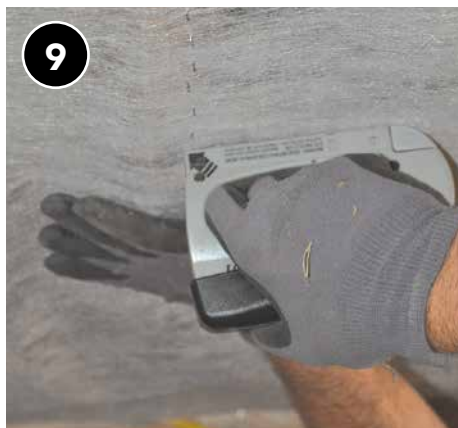
9 For work orders that require netting, secure a smooth layer of netting across the bottom of floor joists.
