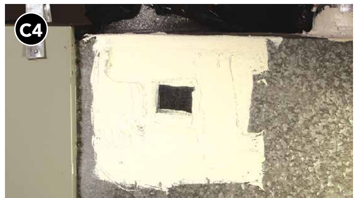
Apply additional mastic over mesh, extending at least 1 inch past tape and seam in all directions.
