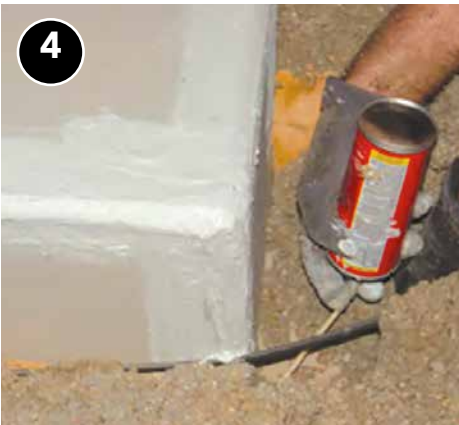
4 Seal box on all sides and edges to make continuous barrier from attic.
