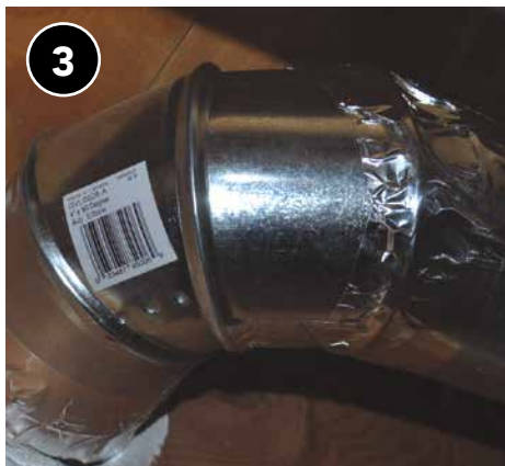
Use correct fasteners (no screws penetrating into duct).
