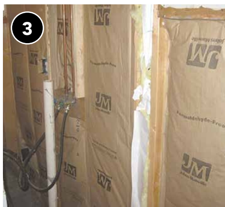
If insulation has vapor retarder on only one side, install the facing towards the conditioned space.
