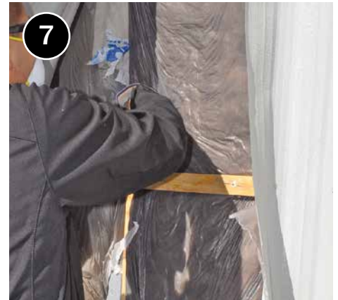
7 Gently tug batt into place, tuck remaining batt under lower belt rail, and fit down to bottom of cavity with minimal compression.
