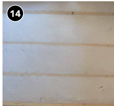
14 Insulation with complete coverage that does not settle will improve the thermal performance of the floor assembly.
