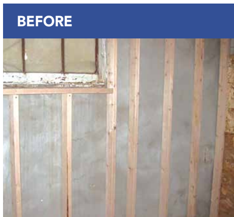
An uninsulated wall in a "conditioned" space allows little resistance to heat transfer.
