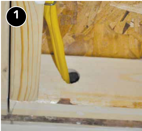
1 Electrical, plumbing, and HVAC penetrations are often oversized.
