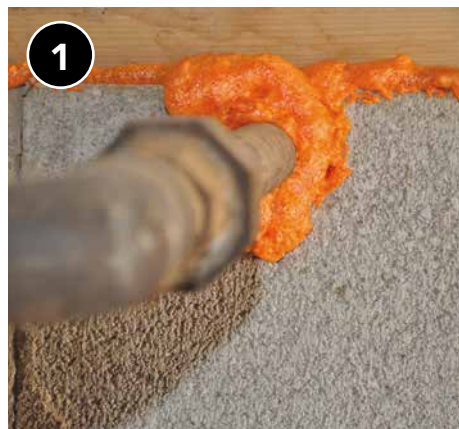
Check the foundation wall for penetrations and air seal as needed prior to installing insulation.
