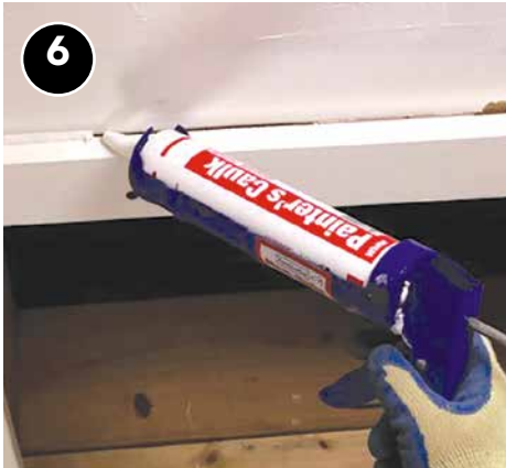
Trim is air sealed with appropriate material.
