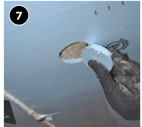
7 Plug access hole either with original material cut out or appropriate replacement.
