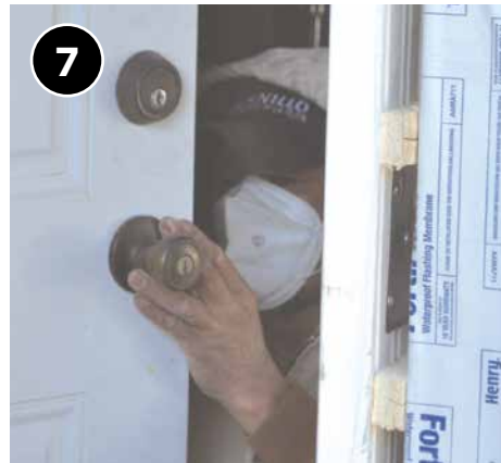
Ensure door is fully operational and lockset is aligned.
