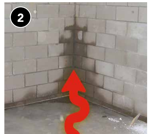
Check wall for water intrusion that needs to be mitigated first. All bulk sources of moisture should be directed away from the foundation walls.
