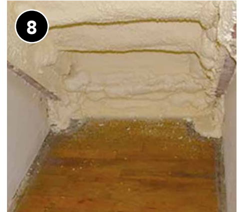
If the stairs have no backing material (e.g., drywall, plaster, etc.) towards the house or conditioned space; insulate with material specified by the work order.
