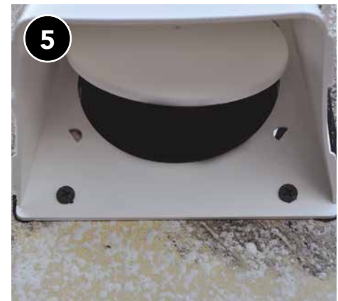
Termination has backdraft damper and no cage.
