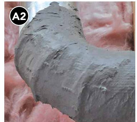
Apply mastic over all mesh tape and all gaps, seams, joints, etc.
