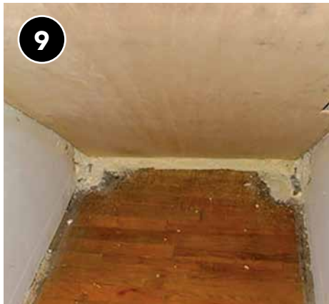
Cover insulation with an approved thermal barrier material for fire safety and to seal off insulation from conditioned space in home.
