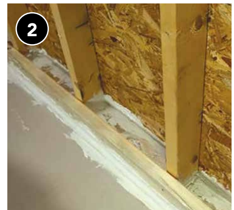
Ensure balloon-framed walls are blocked at top and bottom to prevent insulation from unintentionally blowing into the attic or basement.
