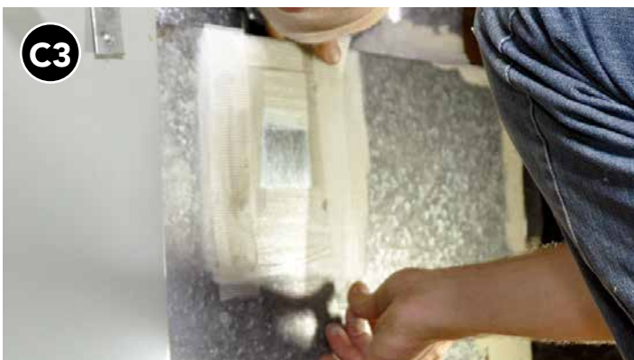
Apply mastic over edges and fasteners of patch and push fiberglass mesh into it.
