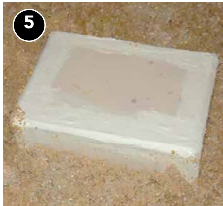
5 Top of box must be R-1 or less and left free of insulation. Flag enclosure for added visibility.
