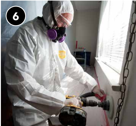
6 Wear appropriate personal protective equipment (PPE), including disposable coveralls, gloves, and P-100 HEPA disposable or fit-tested respirator.
