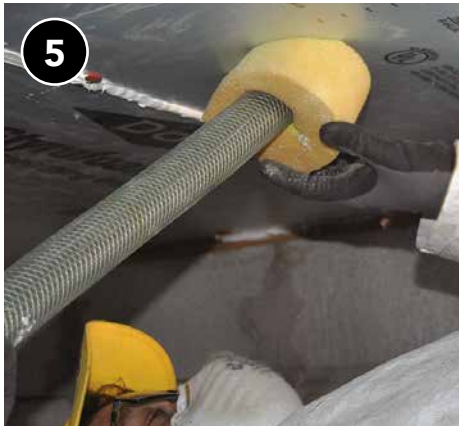
5 Use appropriate fill tube to insulate each cavity and ensure complete coverage.
