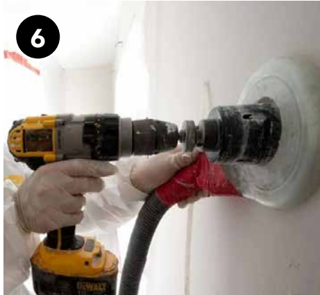
If walls are enclosed from attic side, drill holes in stairway walls defining the thermal boundary.
