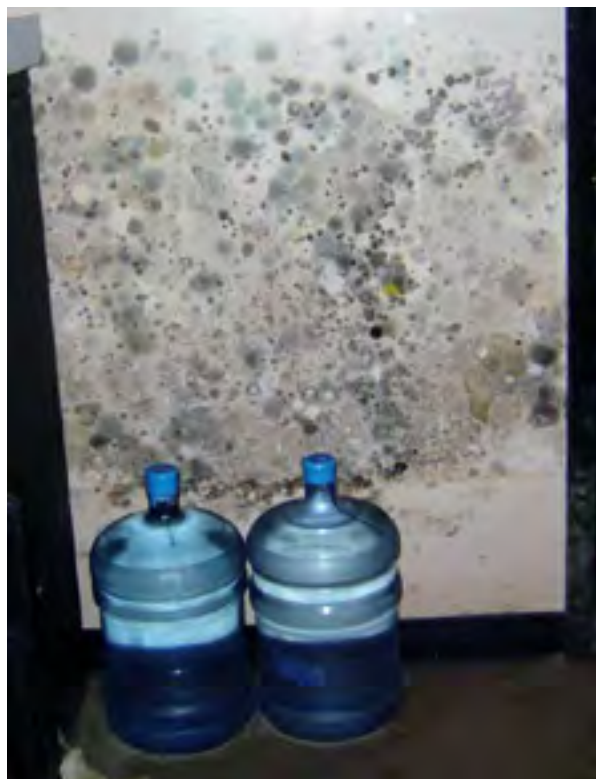
Mold growth on wall board.
