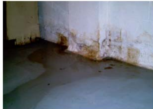
Water damage in the basement.
