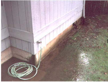
Moisture/ water intrusion
