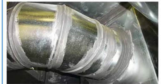
This duct appears to be sealed properly. Leaky ducts can be easily sealed using mastic and/or foil tape.
