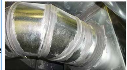
This duct appears to be sealed properly. Leaky ducts can be easily sealed using mastic and/or foil tape.
