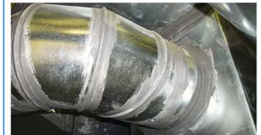
This duct appears to be sealed properly. Leaky ducts can be easily sealed using mastic and/or foil tape.
